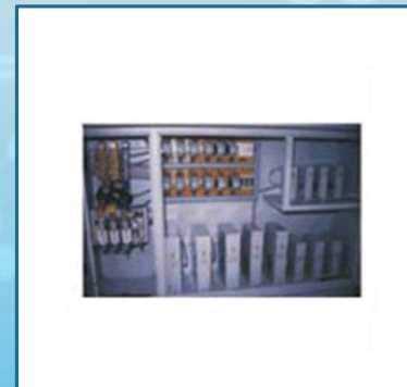
Power Factor Improvement Panel
